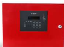
RJV238 Fire Alarm Panel
